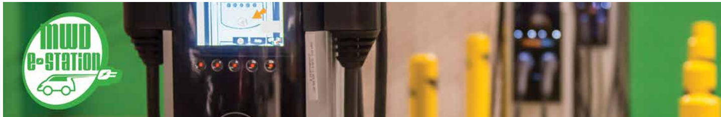
Electric Vehicle Charging Station at MWD Headquarters
