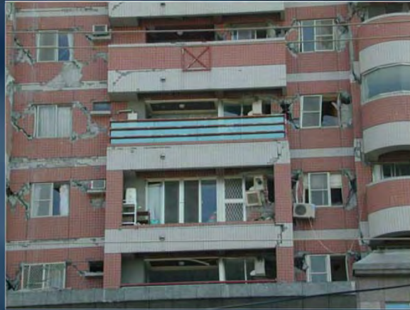
1999 Chi-Chi (Taiwan) Earthquake
