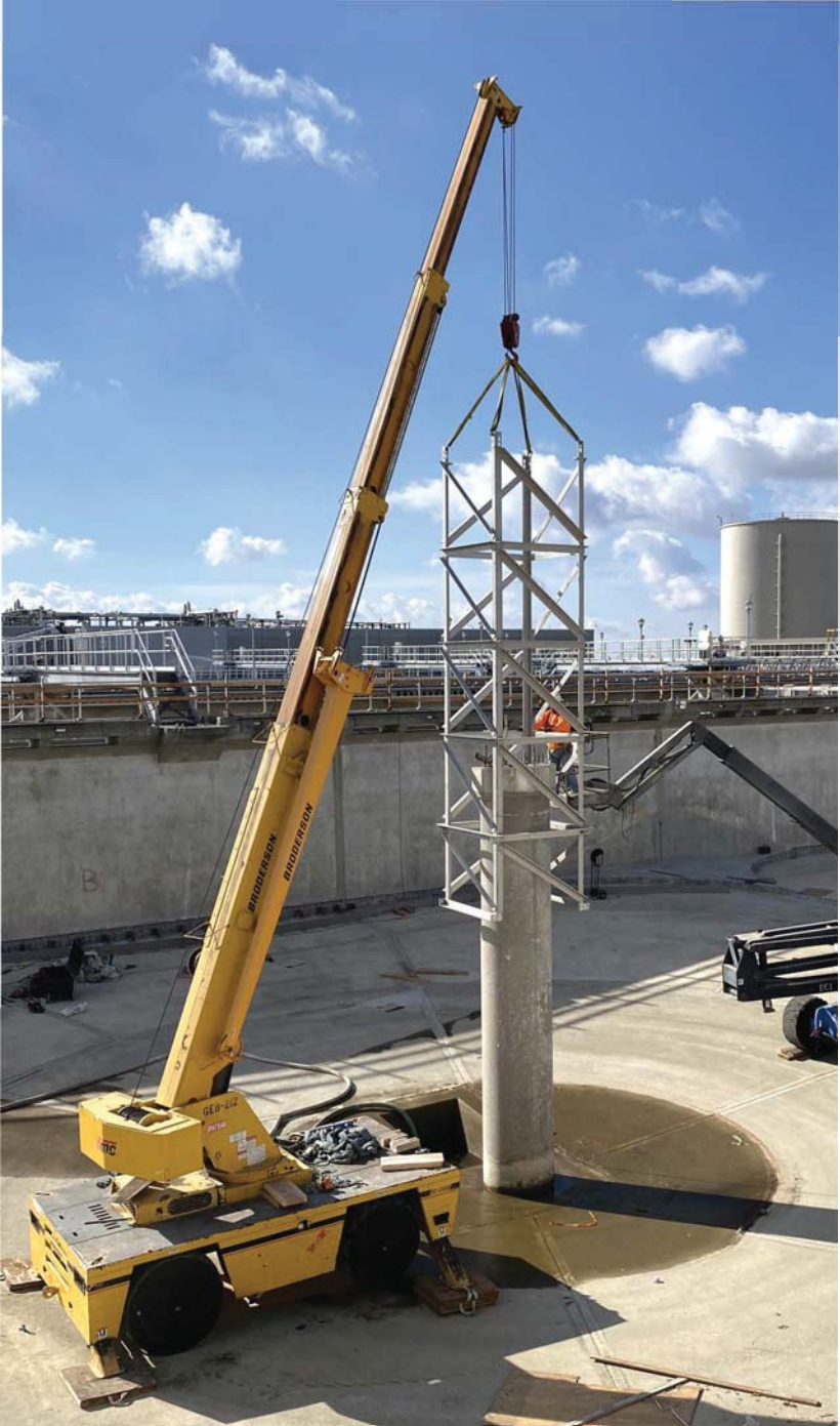
Diemer West Basins and Filter Rehabilitation Project – setting of the turntable support cage in Basin 8.
