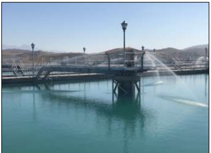
Diemer Plant East Basin No. 3 in operation
