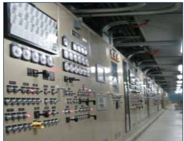
Wadsworth Pumping Plant Pump/turbine control panels
