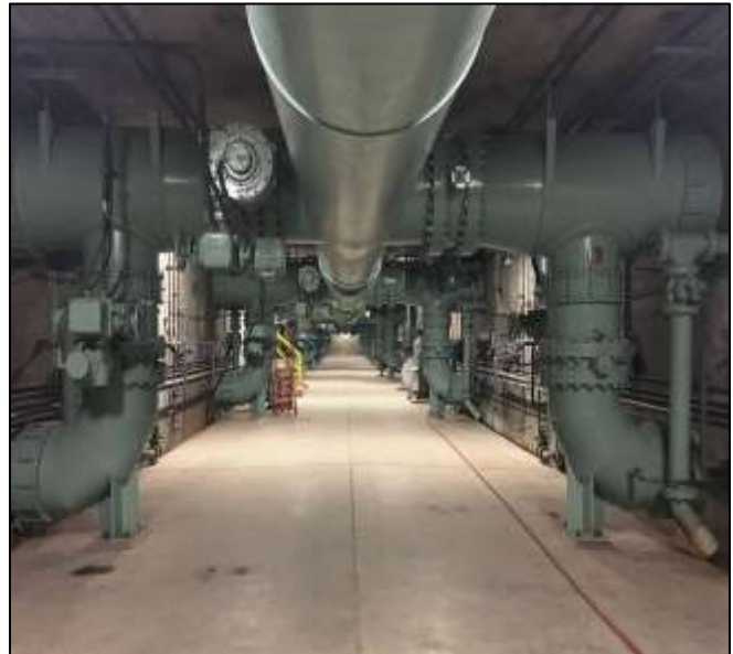
Diemer Plant New backwash and filter outlet valves
