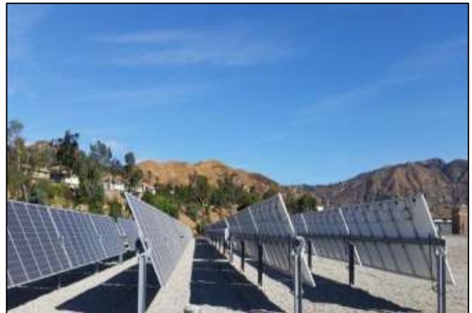
Jensen Solar Power Plant
