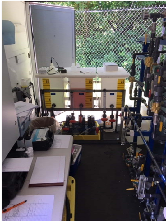
Photo 3. Reagent chemical pumping system
