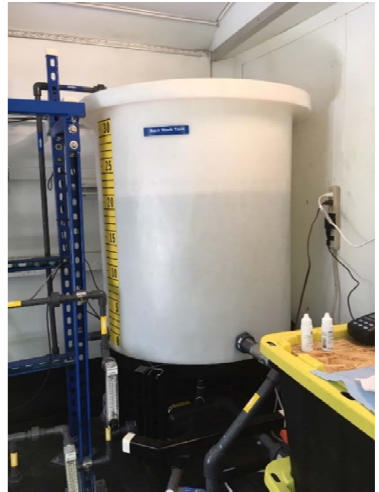
Photo 2. Filter backwash water collection tank.
