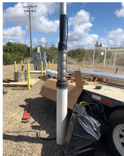
Figure 7-1. Permanent pump prior to installation.
