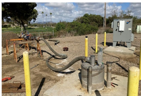
Figure 7-2. Permanent Pump testing.
