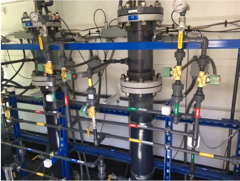
Photo 1. Filter test column units
