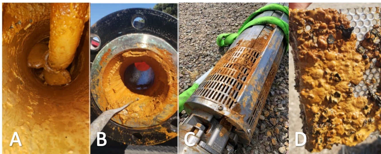
Figure 9-1. Iron and Manganese fouling of the Desalter Test Well. A) Iron fouling of propeller style flow meter. B) Iron fouling deposits in discharge piping. C) Iron fouling on test pump intake. D) Iron (orange) and Manganese (black) fouling on screen located in discharge piping.
