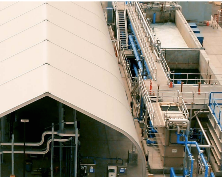
Left: Metropolitan's Regional Recycled Water Purification Demonstration Plant
