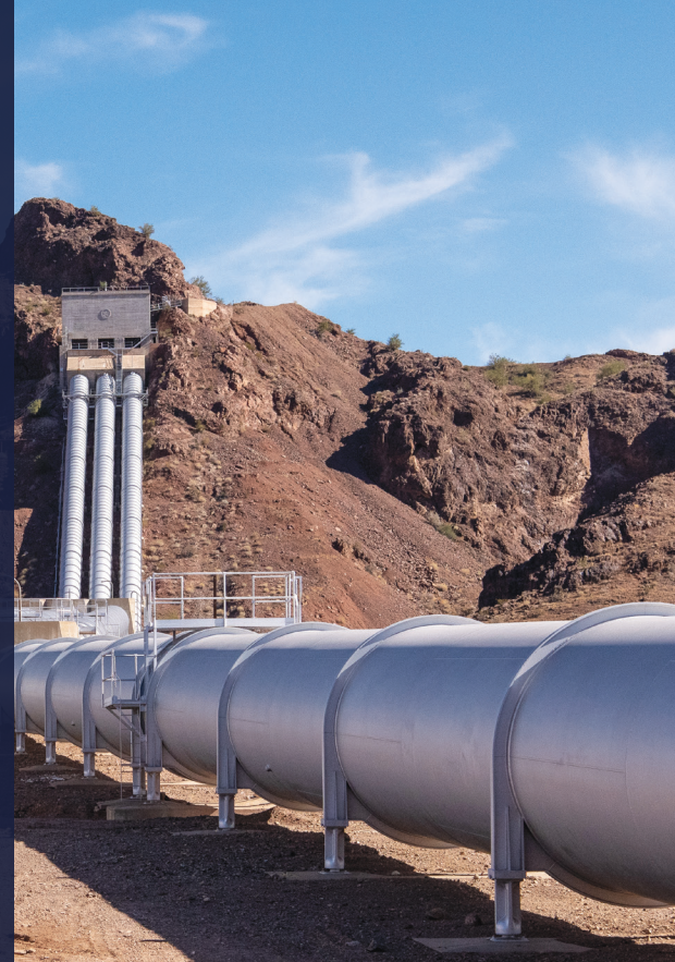
Gene Pumping Plant
