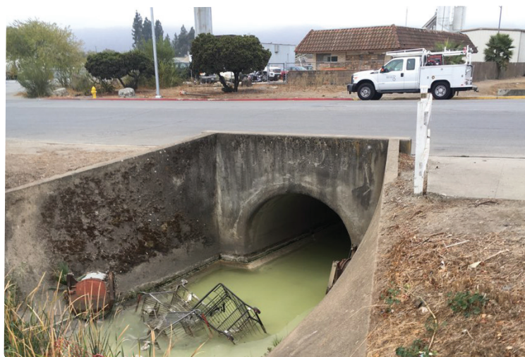
Princeville Drain (Gilroy) received contaminated discharge from nearby source.
