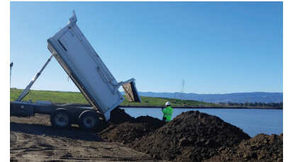
Sediment delivery to Pond A8.
