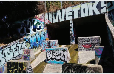
Graffiti located on the energy dissipating drop structure in Lower Silver Creek at Tuers Rd. in San José.
