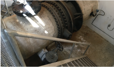
Shannon line valve.
