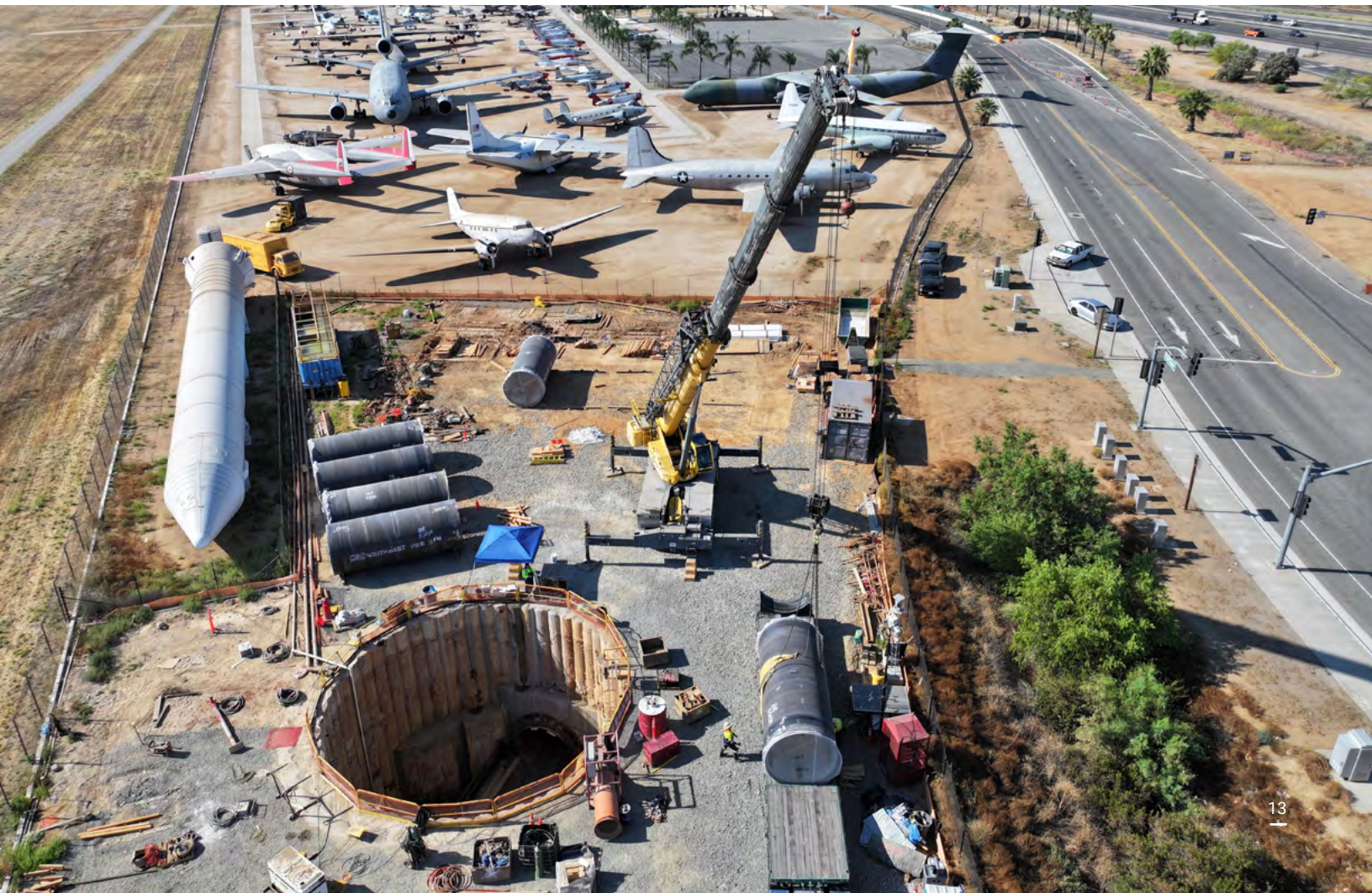
Shaft for Perris Valley Pipeline I-215 Crossing near March Air Reserve Base
