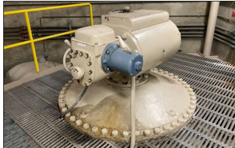
Valve Inside Junction Structure Vault.
