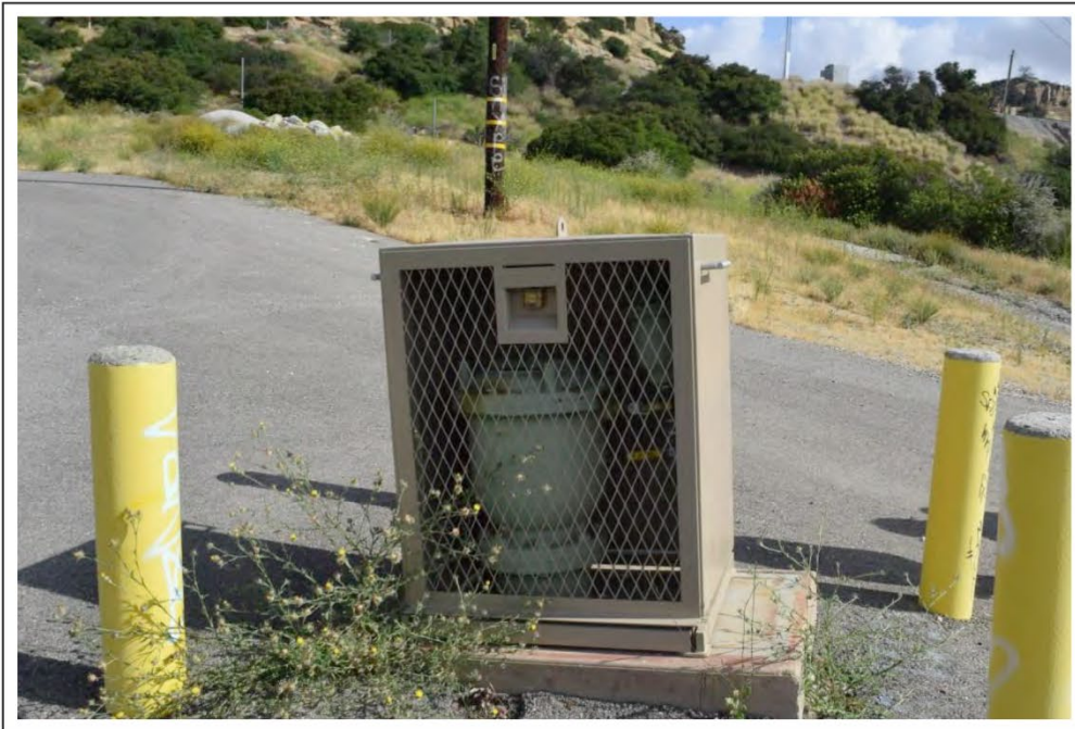
WWF1 Station 1405+23, Air Release and Vacuum Valve enclosure, facing north.
