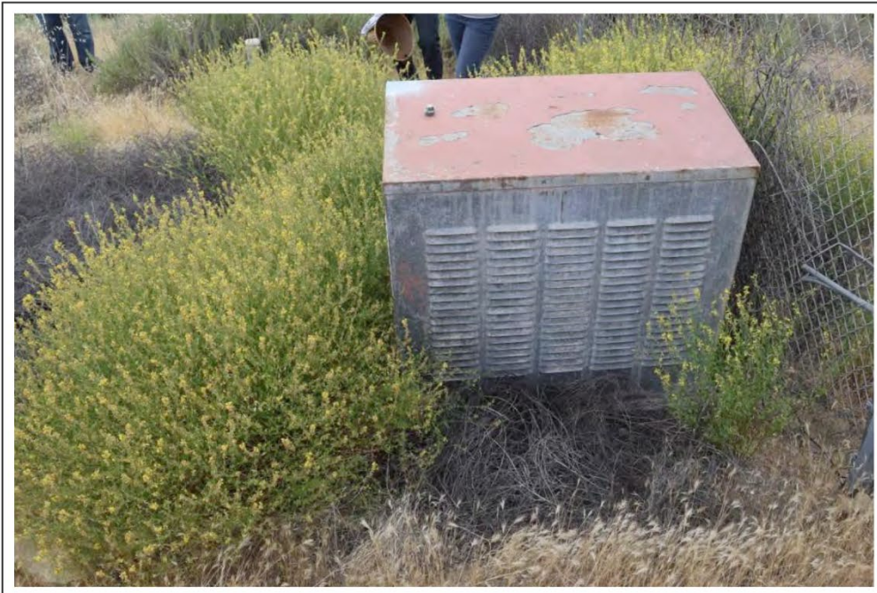
WWF1 Station 1415+37 and 1415+42, Air Release and Vacuum Valve enclosure, facing south.
