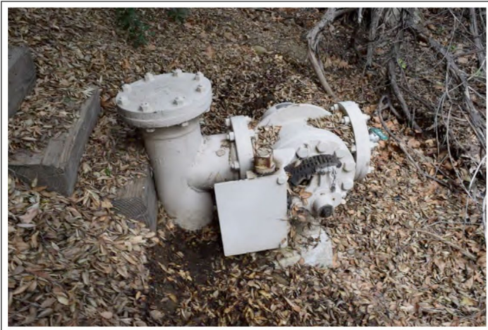
WWF1 Station 1416+33, exposed valve, facing north.
