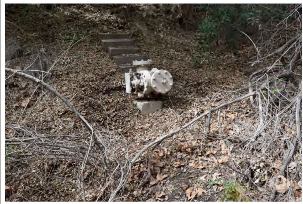
WWF1 Station 1416+33, exposed valve, facing west.
