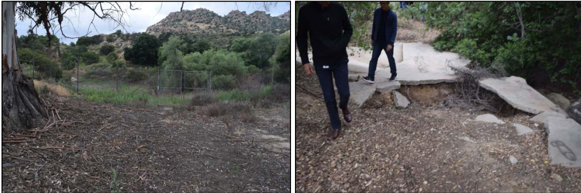
Figure 4 - Earthen Flood Control Basin and Broken Spillway
