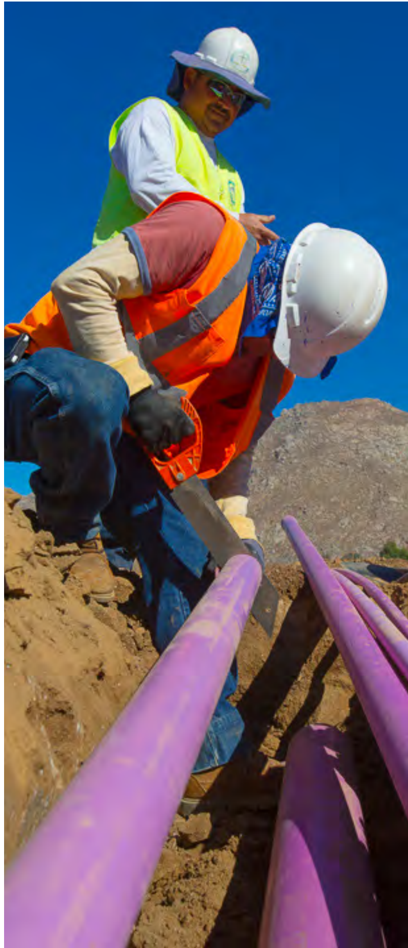
Installation of recycled water irrigation lines with support from the Local Resources Program
