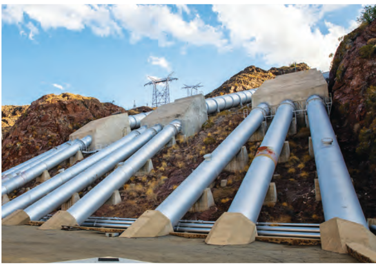
Whitsett Intake Pumping Plant
